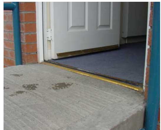
Figure 1 A level threshold is where the external walking surface is level with the door threshold and the internal floor finish
