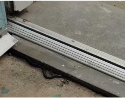
Figure 16 Screw fixings left proud of the threshold unit, as a result of repair, could be a trip hazard
