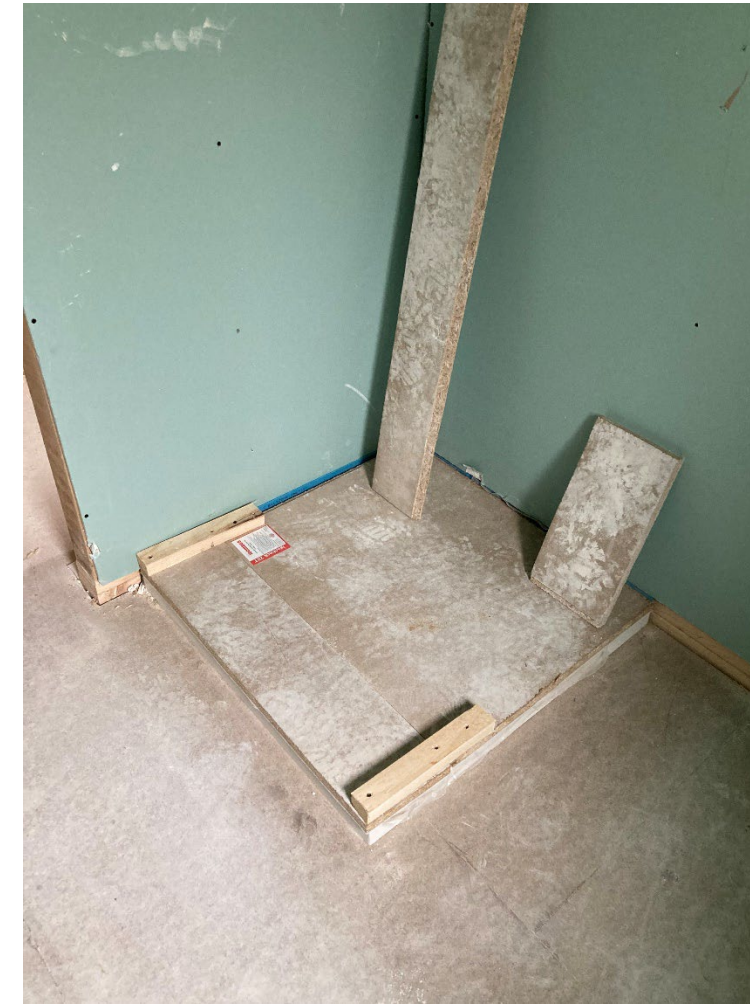
Requirements for step in access shower trays as flush shower trays have structural, fire, and sound issues
