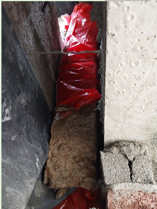
Damaged materials No longer fit for purpose
