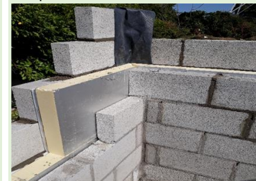
September 2018 Mock-up. Adequate wall tie installation, vertical DPC installed to external corners, full fill cavity.
