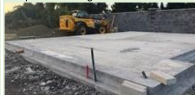
Photo Above; September 2018 Blockwork entirely deconstructed back to ground floor slab level and arisings removed to a licensed waste facility.
