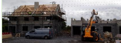
Photo Above; August 2018; Partially constructed houses, roof timbers complete to first set, with blockwork approaching completion on second set.
